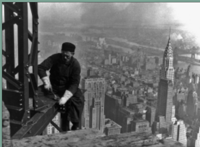
A workman on the Empire State Building in New York City, 1930, by Lewis Hine. (69-RH-4K-1, Washington, DC)
